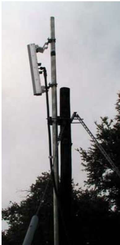
XM repeater panel antenna - photo courtesy Frank Martin
